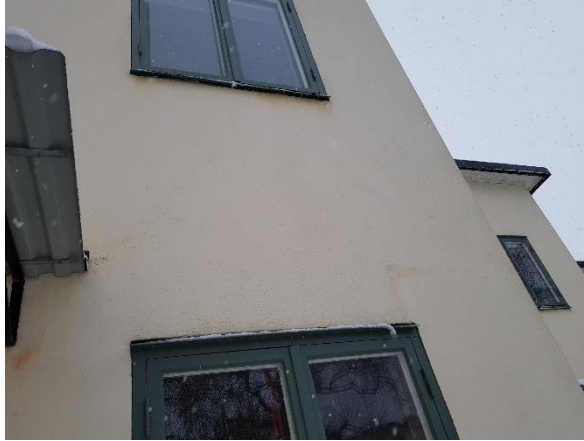
Figur 2. Fasad i ok skick.
